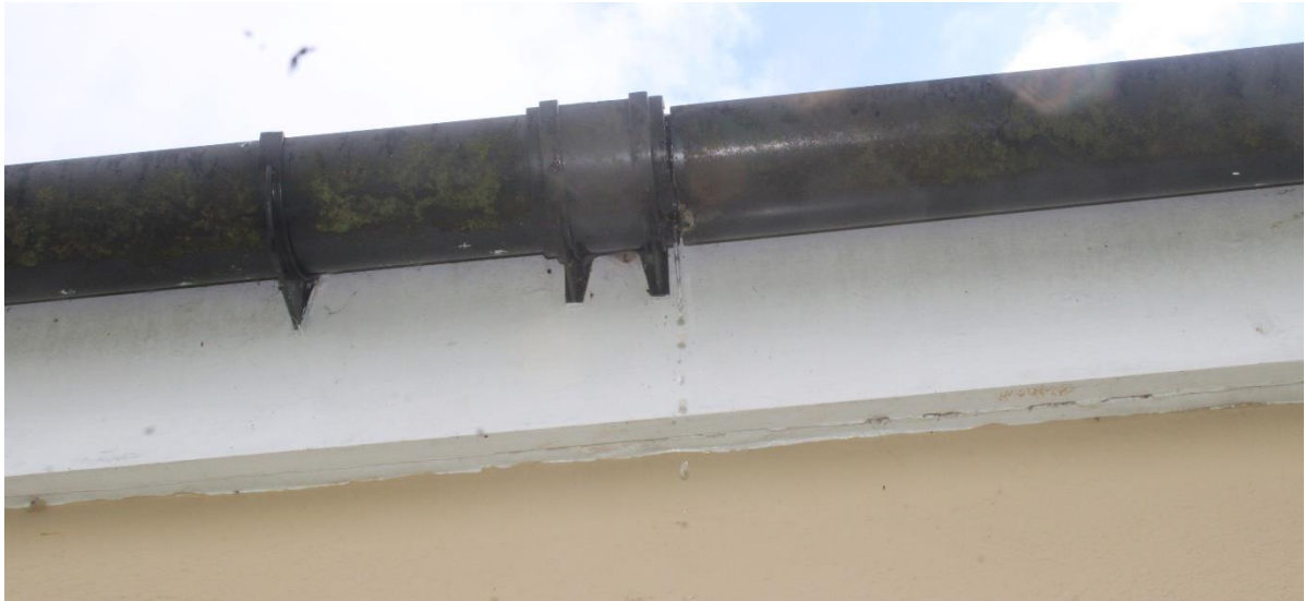
Leaking plastic gutter.
