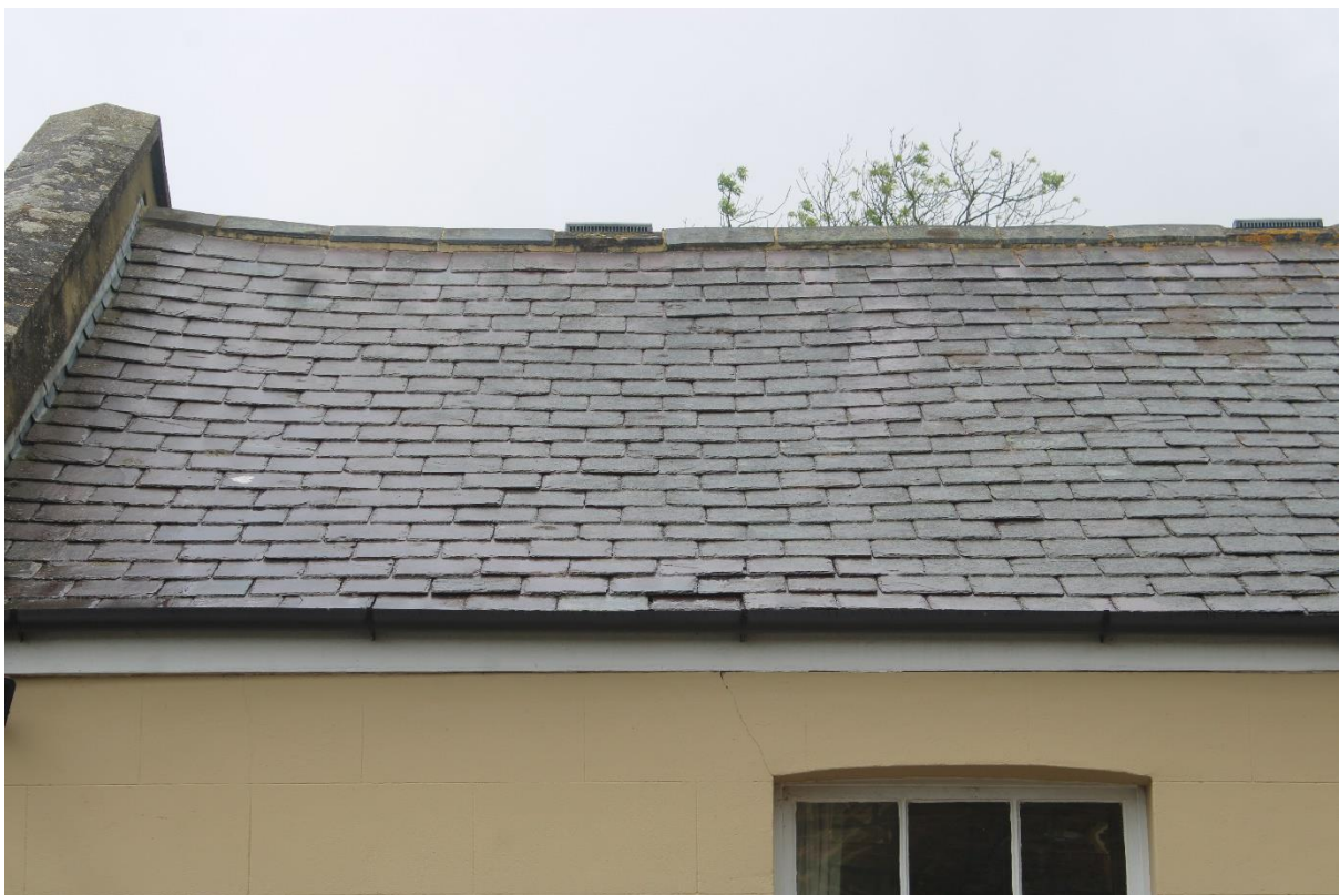
Roof surface: note parapet upstand, slight sagging, vent tiles set along ridge and fascia board fixed tight to wall.
