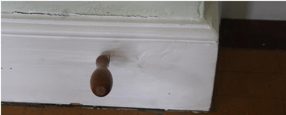
Decayed section of skirting to wall between kitchen and main hall.
