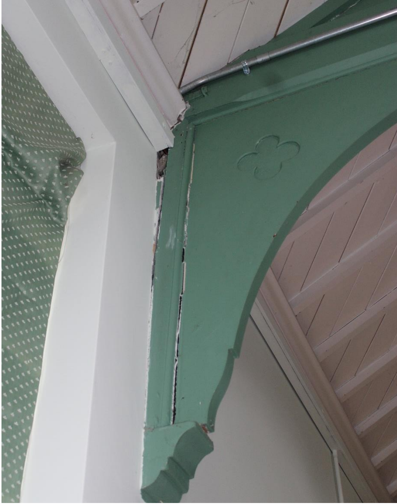
Open joint to side of post and wall and spandrel panel to one of the trusses in the main hall.
