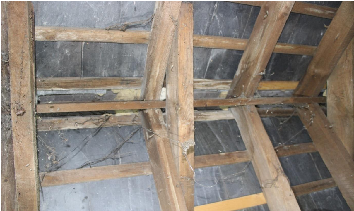
Underside of roof: note no underlay and damp staining to timbers.
